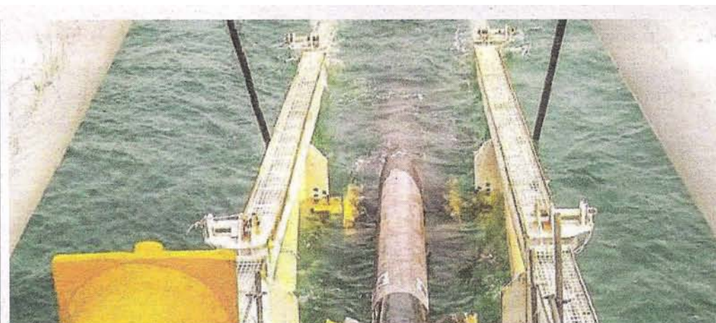
Alam Maritim's jointly-controlled Alam Swiber Offshore has secured a contract from Chevron for the installation works for the replacement of subsea pipelines at the latter's Prai Terminal.
